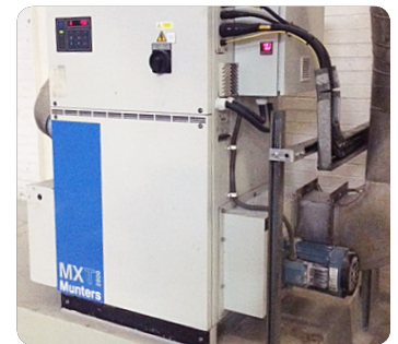
Before upgrade A Munters MXT2800 dehumidifier equipped with the original fan
