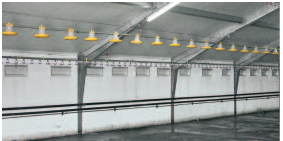
Several IW Air inlets mounted into a poultry house.
