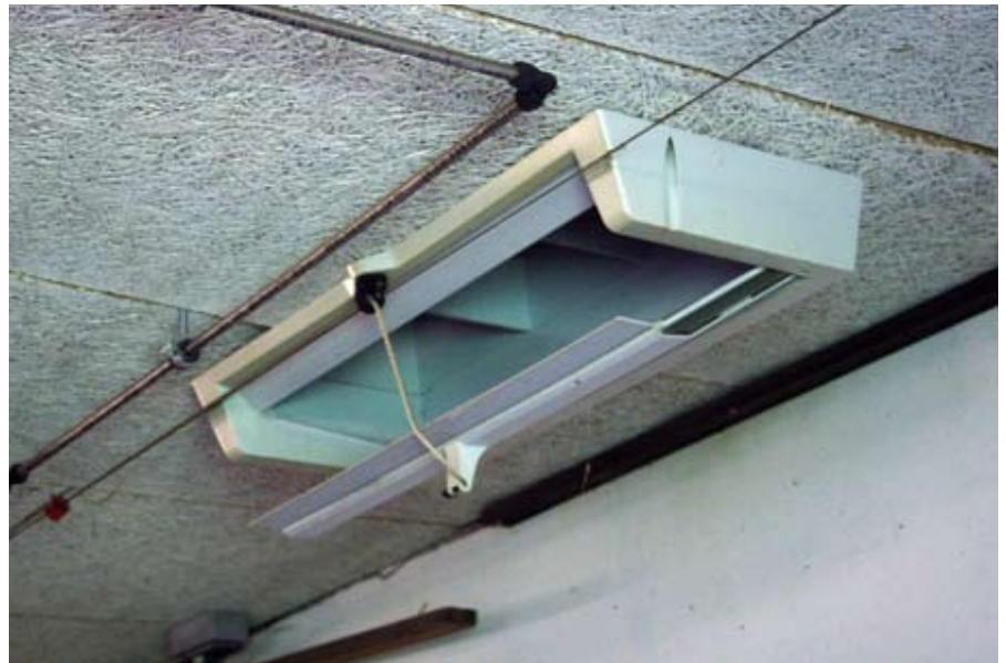
IL Air Inlet mounted into a swine house.
