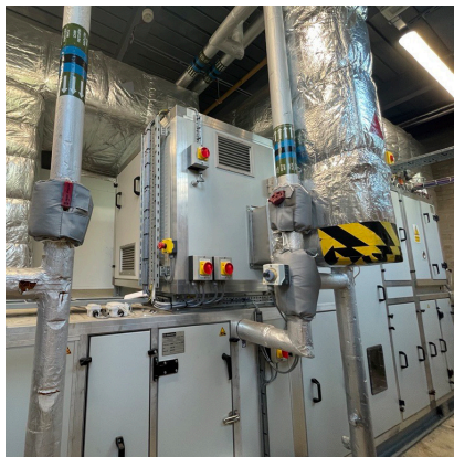
The Munters desiccant dehumidification system installed in the plant room.
