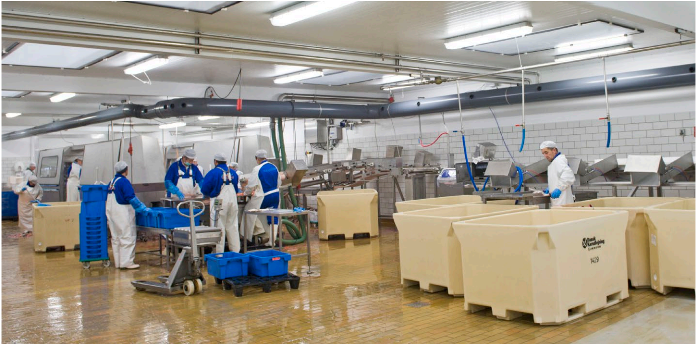
Despite the use of huge amount of water during processing, the ceiling is free of condensation after installation of Munters dehumidification system.
