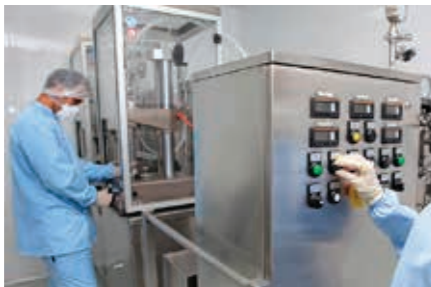
2. Cleanroom & R&D Everything in a cleanroom needs to be accounted for and within specification, and that includes the air. Without proper humidity control, the exterior climate can affect the room conditions.
