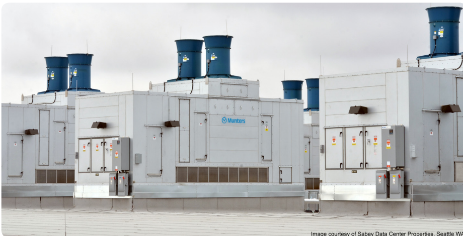
Image courtesy of Sabey Data Center Properties, Seattle WA
