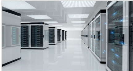
Data Center cooling solutions
