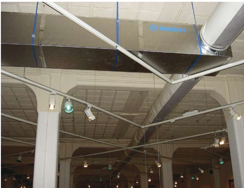
Insulated main air duct, with perforated hoses give good air distribution.
