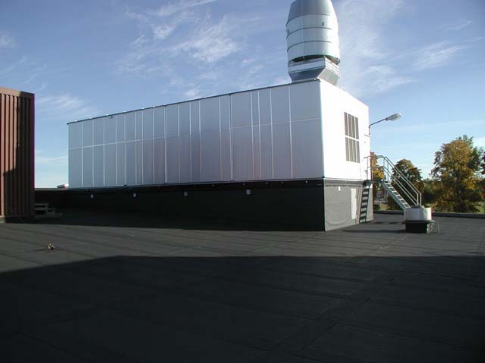
Munters environmentally friendly DesiCool Systems installed at Sandvik Tools facility
