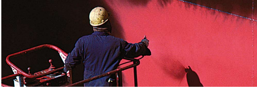
New paint is applied in several layers to the clean steel structure.
