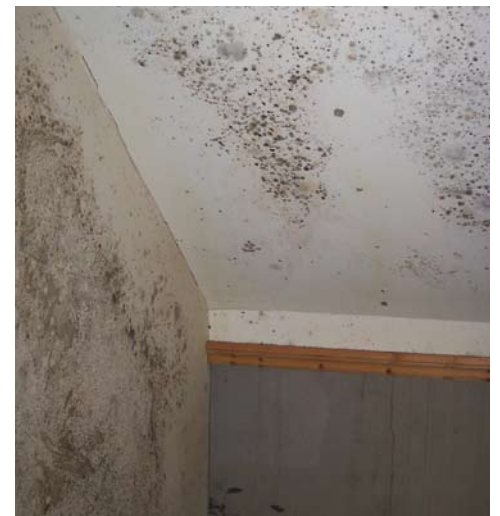
Mould contaminated plasterboarding.
