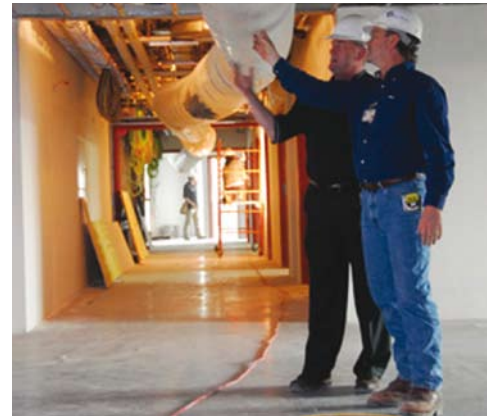
Temporary plastic ducting is utilised to effectively distribute treated air to all areas of the project site.
