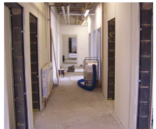
Munters units in position.
