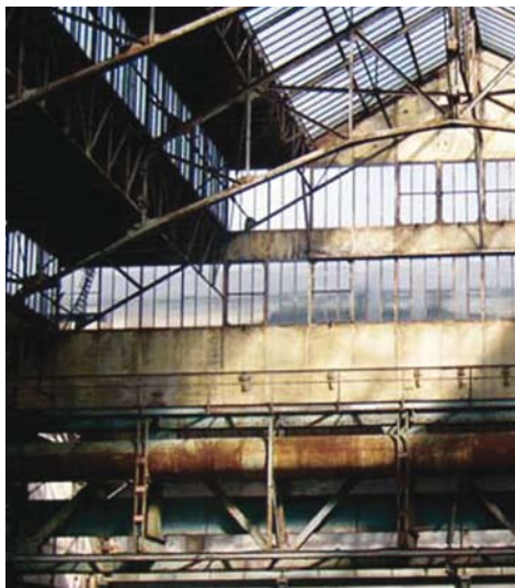
Structure requiring cleaning.
