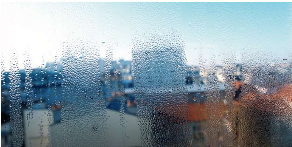
Poor building efficiency can result in damaging condensation.
