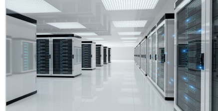
Data Center cooling solutions
