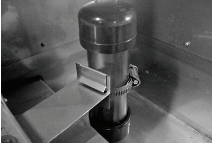
Figure 4.6 Chloride tablet dosing system
