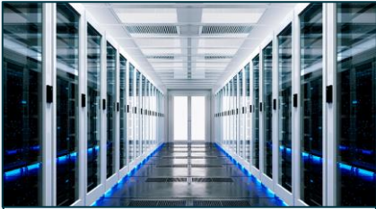
Cooling solutions for Data Centers
