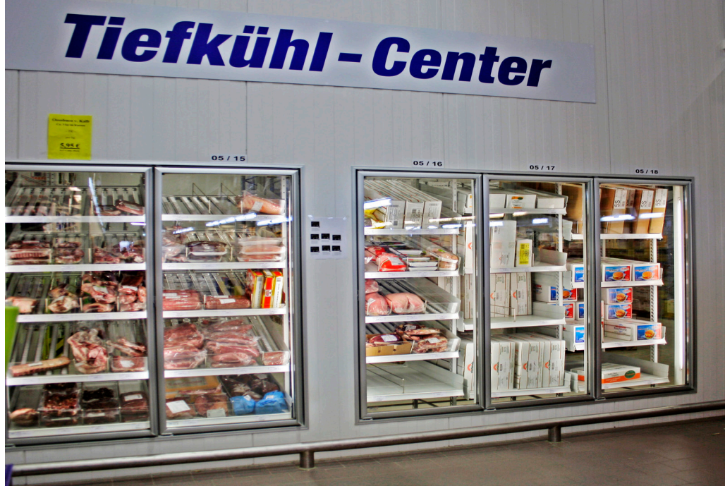
The employees working in the -15°C cold store enjoy safe working conditions with dry floors free of ice, no formations of fog or ice build-ups on doors, products and ceiling.
