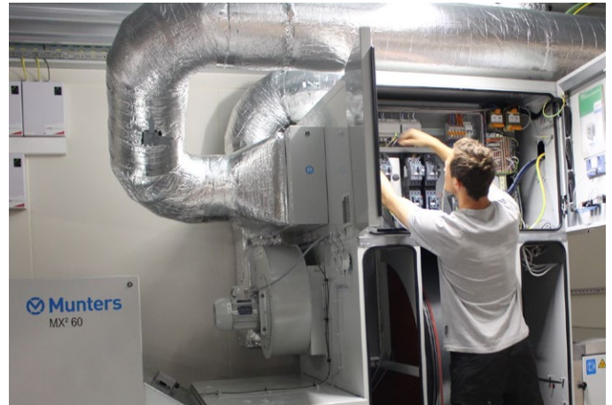
Munters service engineer sets up the MX 2 60 at Kenis Bakery.
